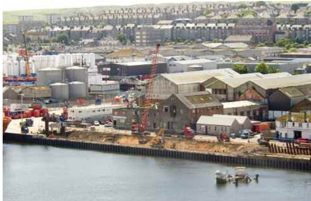
Reconstruction of Albert Quay West, with buildings beyond to be cleared for 20,000 square metres of surfaced back-up area.
