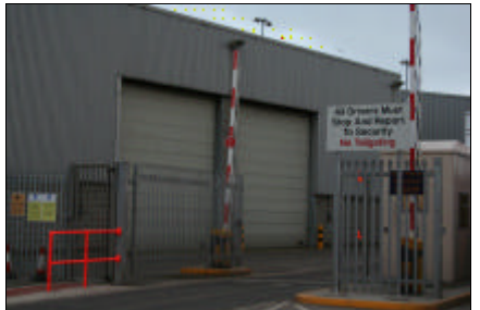
Central Roadway traffic barrier has been struck and damaged on numerous occasions.
