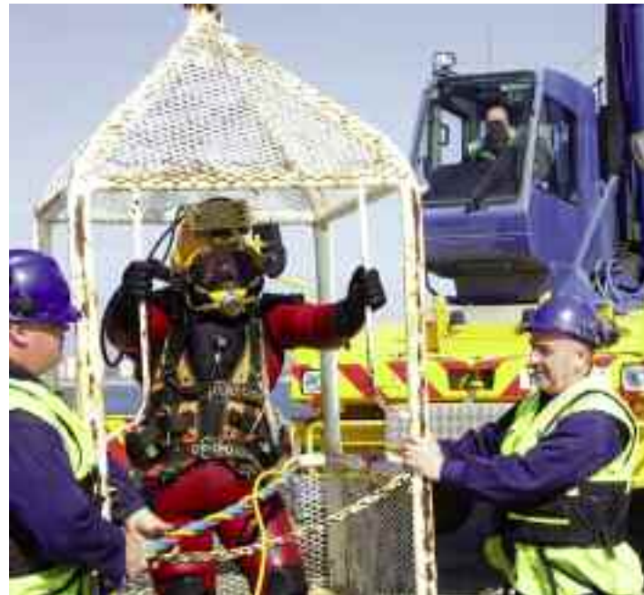
Crane driver, George Buchan, chargehand, Glen McIntyre (left) and labourer, Gordon Dalgarno, prepare a diver for maintenance work.
